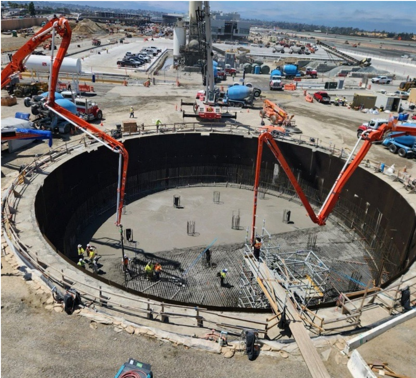
The Airport's new approximately one-million-gallon stormwater cistern captures water for reuse, while new infiltration beds and basins installed as part of NT1 manage runoff through onsite infiltration.
