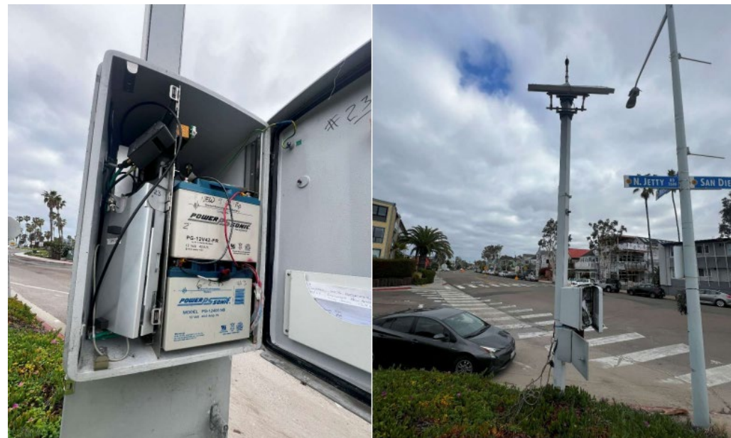
Noise Monitor #23, located in Mission Beach, undergoing maintenance and inspection.
