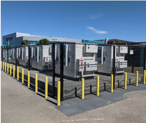
Figure 8: SAN’s 2 MW Battery Energy Storage System.
